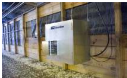
Forced air furnace
