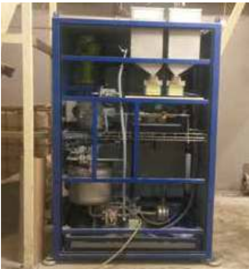
One of the installed Huvematics.
